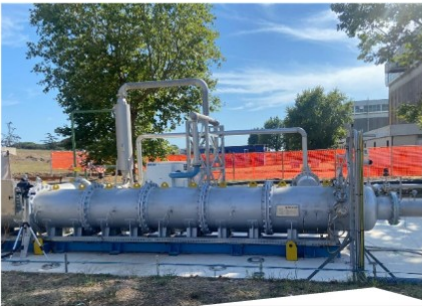
TEMPRA pilot unit -Castel Romano-Italy
