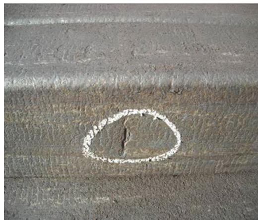
Fig.7 - Cracks with powder entrapment.
