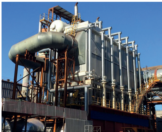
Fig. 4 - Corner Tube Boiler
