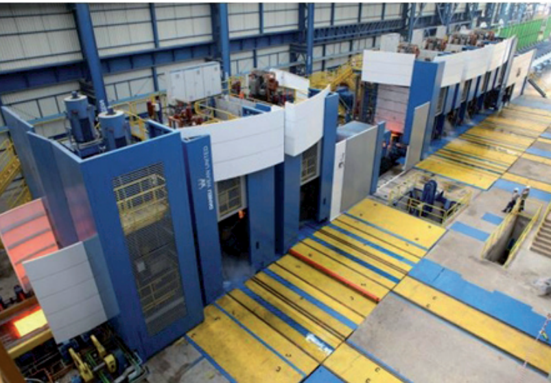
Fig. 1 – Typical QSP hot strip mill configuration.
