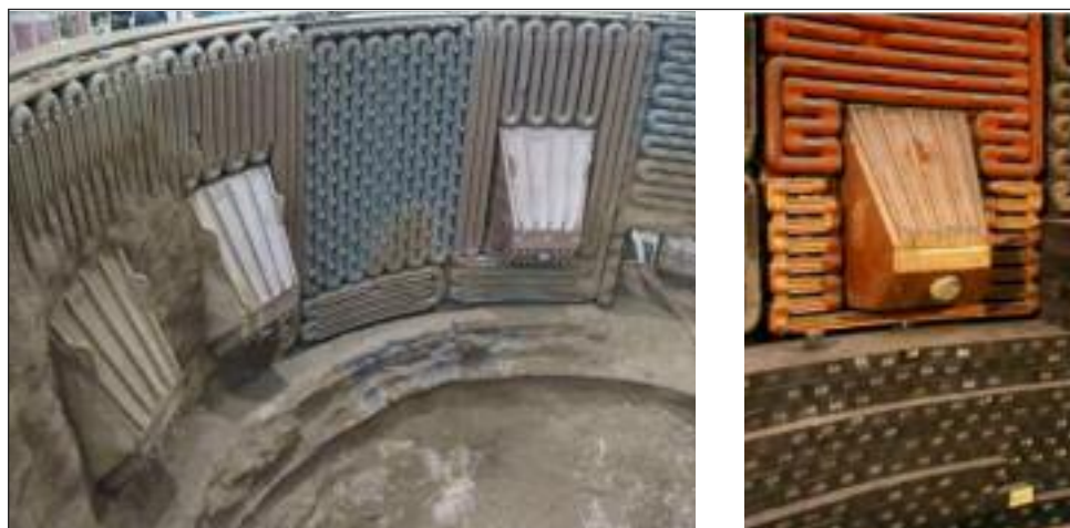
FIG. 3 Bulged panels. Cassoni in rame.
