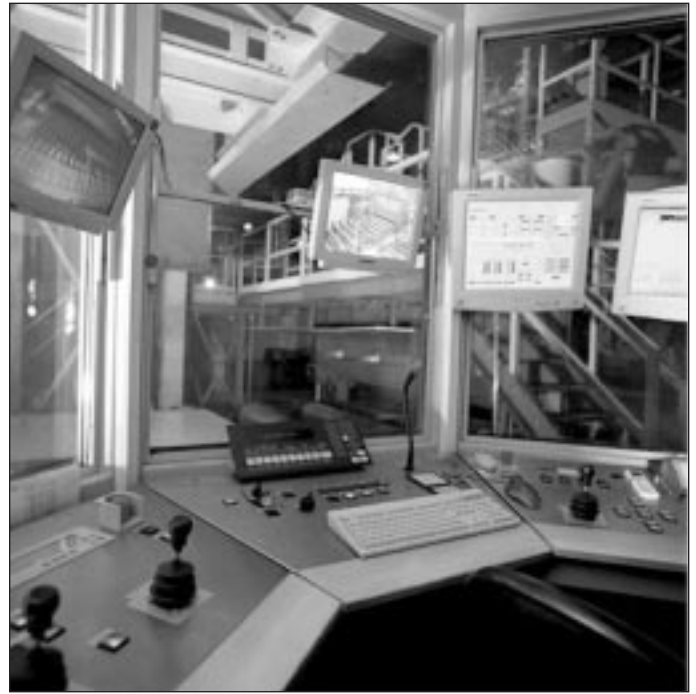
Figure 9: Main Control Pulpit of Plate Mill, Voestalpine Grobblech, Linz, Austria.
