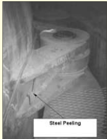
Figure 8: Peeling of Solidified Steel Off of a Horizontal Link Assembly After a Burn-Through.
