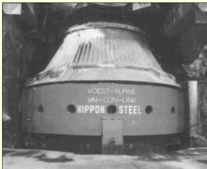
Figure 4: Inspection of the VAI-CON® Link Suspension System at ISPAT ISCOR Newcastle, South Africa.
